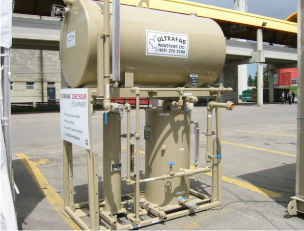
Vent and Instrument Gas H2S Treatment
